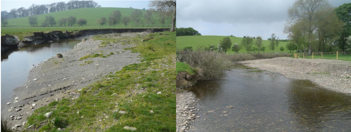
Figs 10 and 11 Garth Dulas at Dolderwen before and after bank protection with timber (and increasing cover) and fencing.
