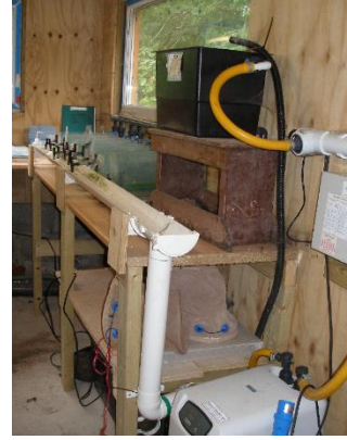
Figure 15. Recirculated rearing system
